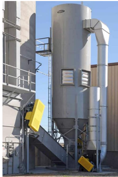
Explosion Relief Panel - Silo
