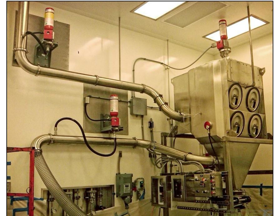
Explosion Suppression System
